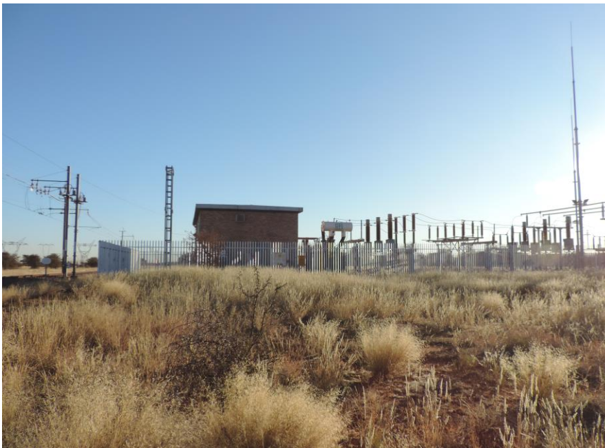
Figure 16 The Emil Traction Substation on the Remaining Extent of the Farm Fritz 540
