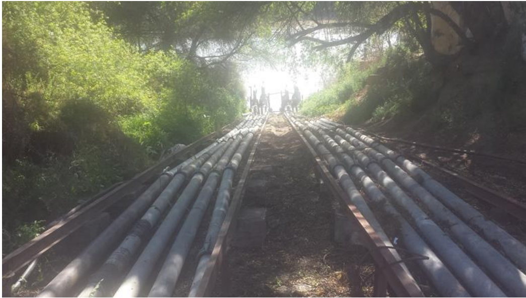
Existing water extraction point in the Orange River
