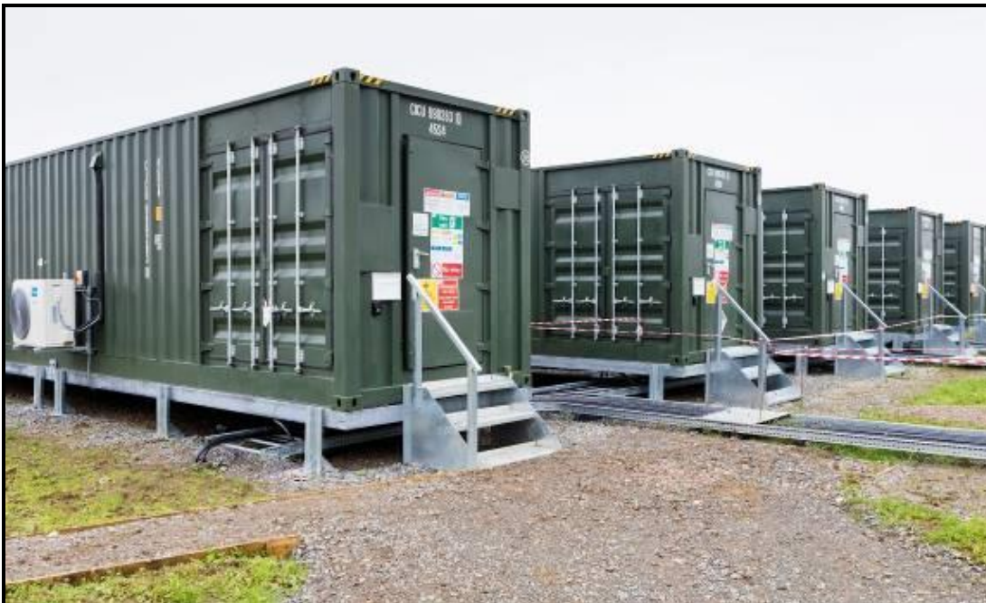
Photograph 1.2: Example of BESS located in storage containers
