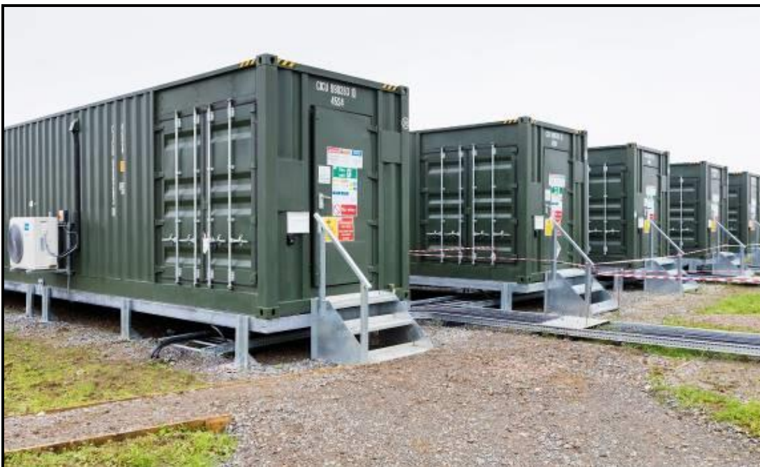
Photograph 1.2: Example of BESS located in storage containers
