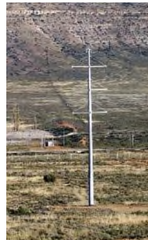
Plate 3, Eskom 220kV Monopole.
