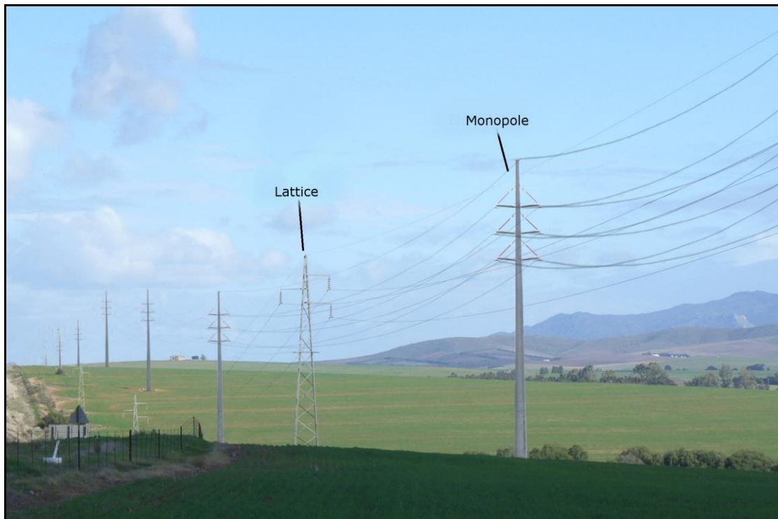
Figure 9: Examples of 132kV overhead power lines.
