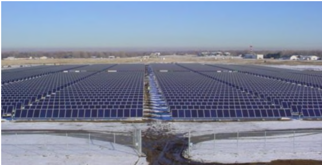
Plate 15 - PV array viewed from above. Note the array rows are read as one and have a similar impact as the roof of a large industrial building.
