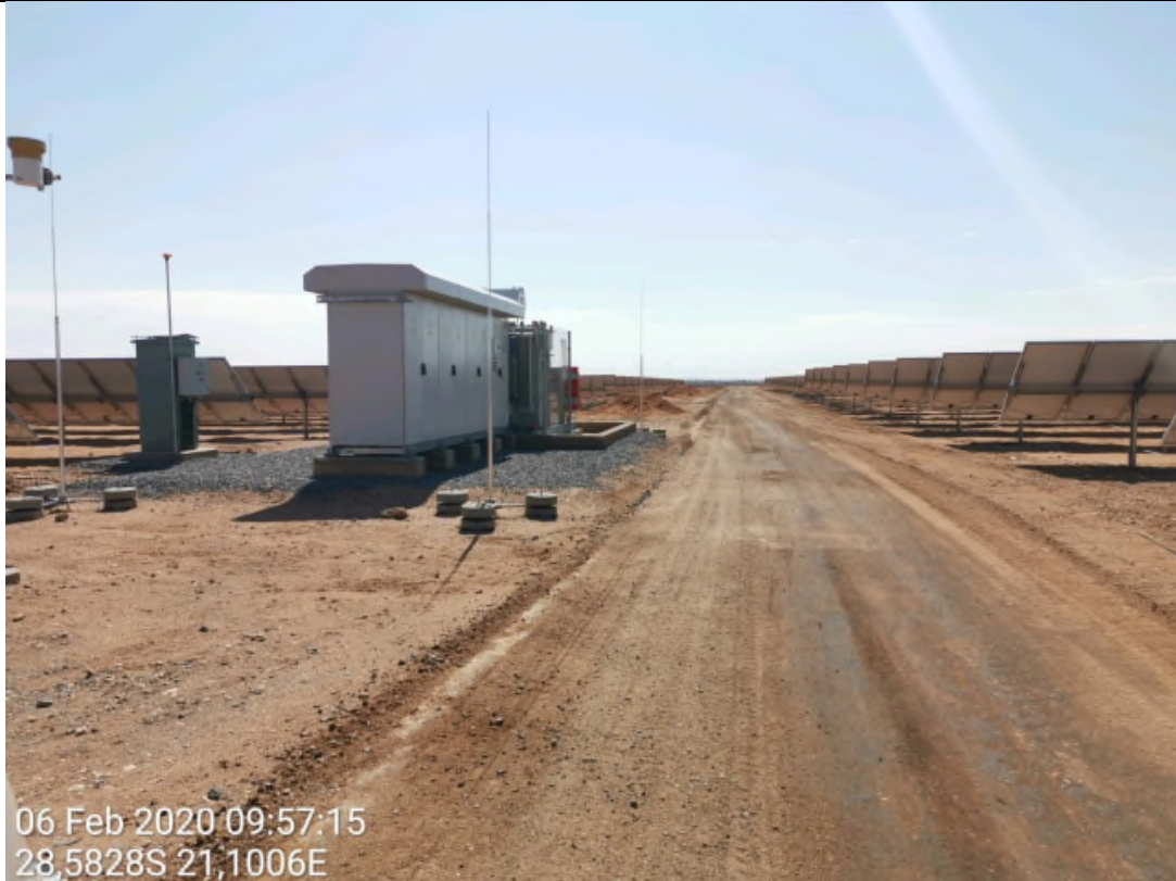
Plate 2, View of tracking PV array with central inverter station in the foreground.
