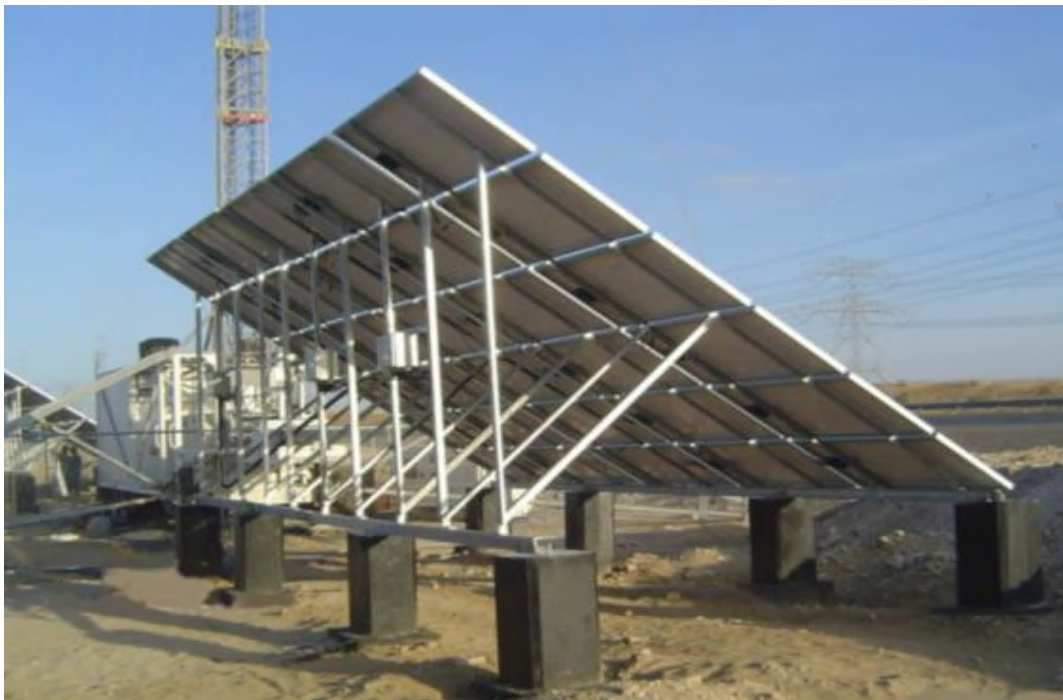
Plate 16 - PV array viewed from behind and the side. The dark face of the PV units are not obvious and subject to the colour of the undersides of the units, the supporting structures are likely to become more apparent. This might appear as a long industrial structure from close quarters. From a distance however, the shadow cast by the structure will be read and will probably appear similar in nature to the front view of the array.
