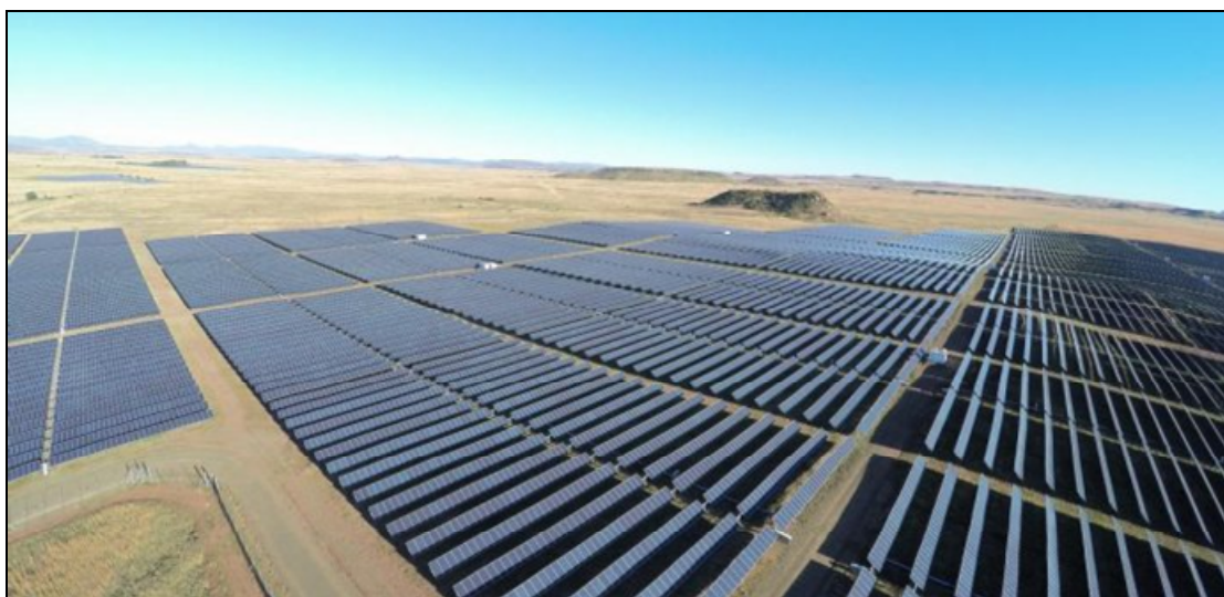
Figure 2: Aerial view of PV arrays. (Photo: Scatec Solar South Africa ).
