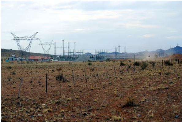
Plate 5, Industrial Landscape Character Area. Paulputs Substation.
