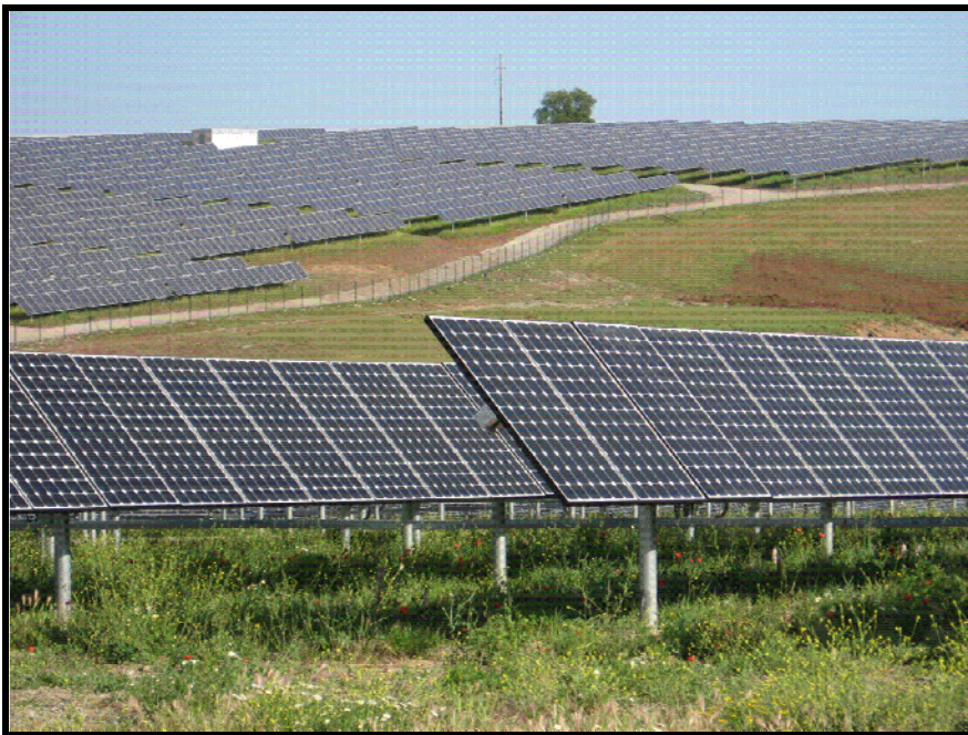
Figure 1.2: Stationary solar PV panels.
