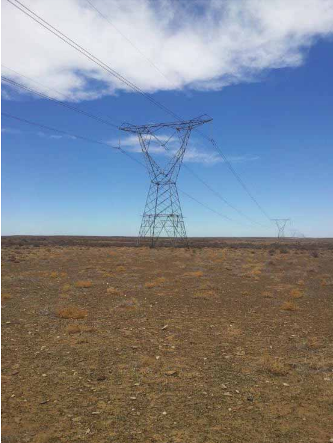
Photo 4.3 Photograph showing a typical electrical power line found throughout the area
