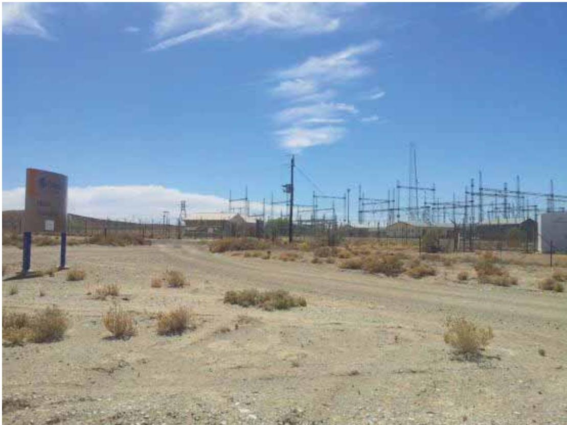
Photo 2.1 Eskom Helios Substation
