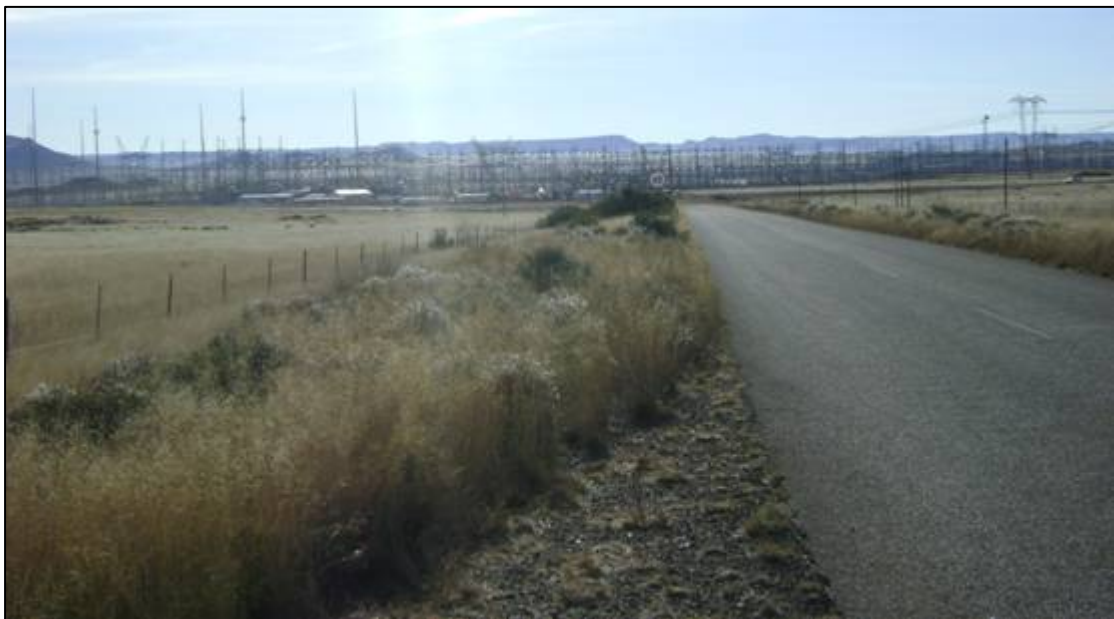
Figure 3: The hydra substation in the south of the study area.
