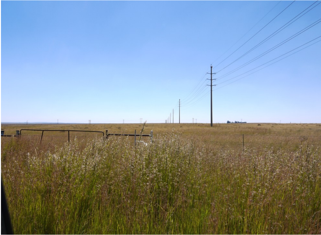
Plate 16 - A view along the line of a 132kv overhead power line with monopole towers
