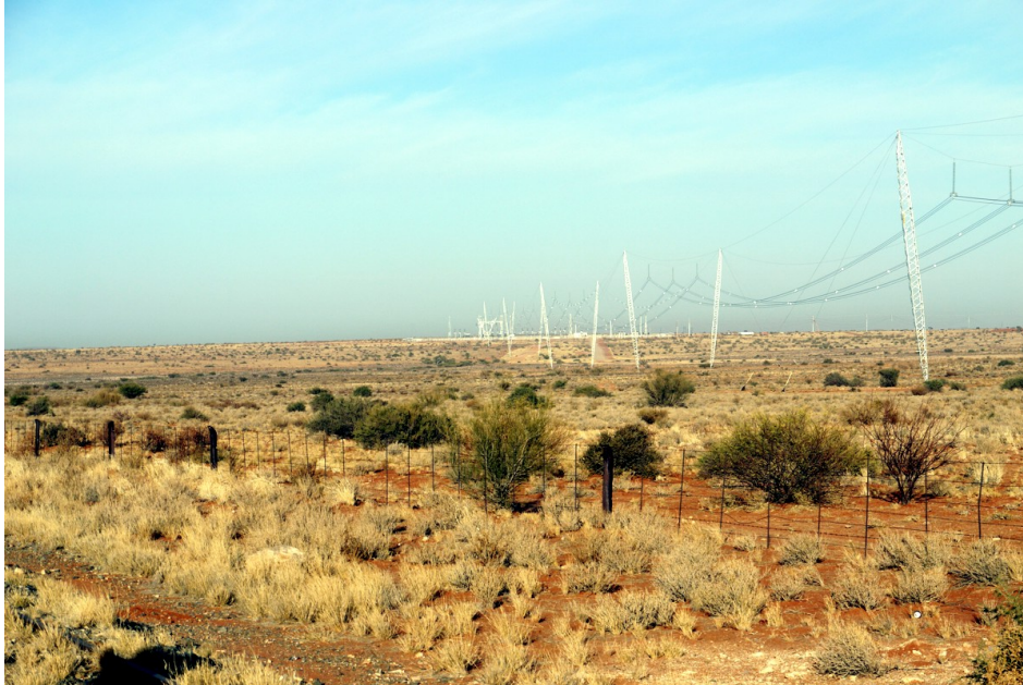
Plate 1, Existing Upington Main Transformer Substation (MTS). Note the Strategic power line connections linking to the Upington MTS
