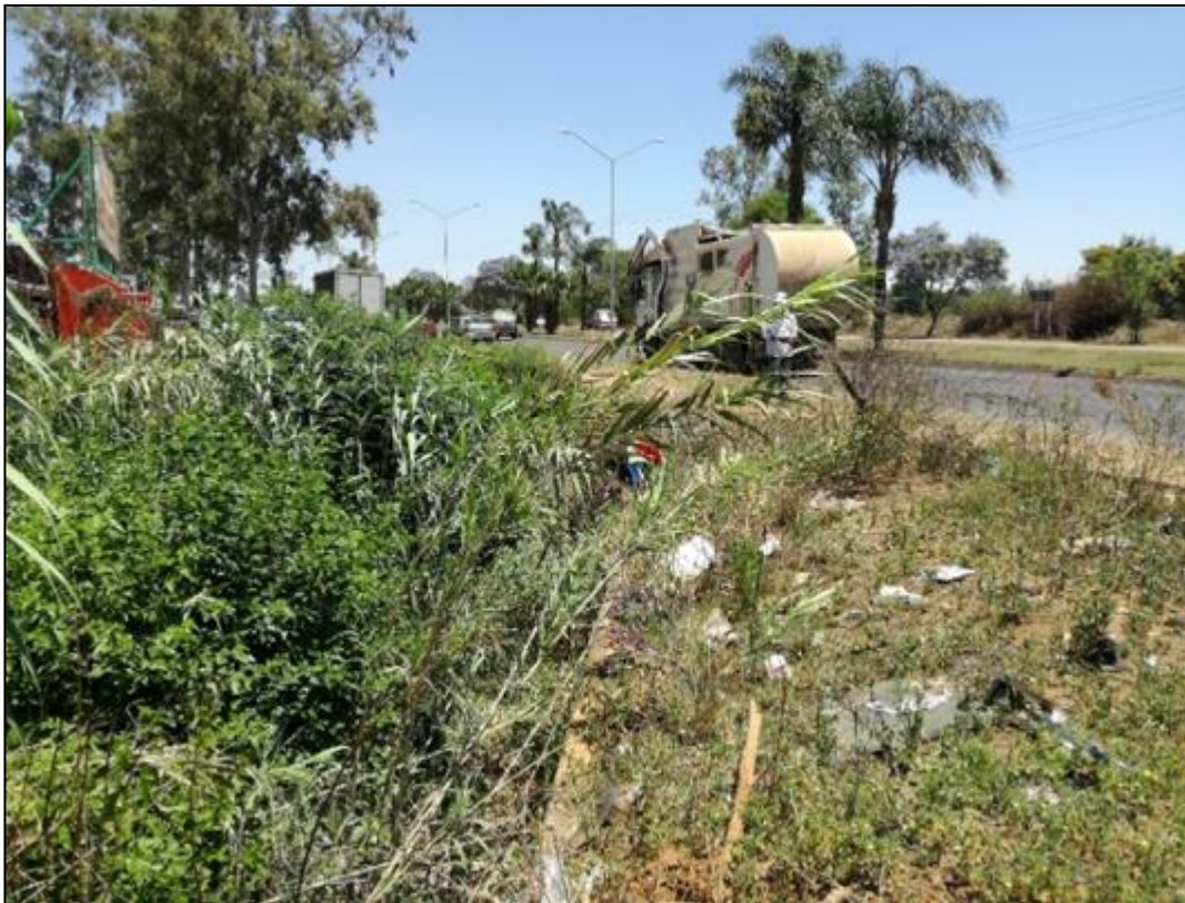
Figure 5: Vegetation Overgrowth at Culvert Entrance
