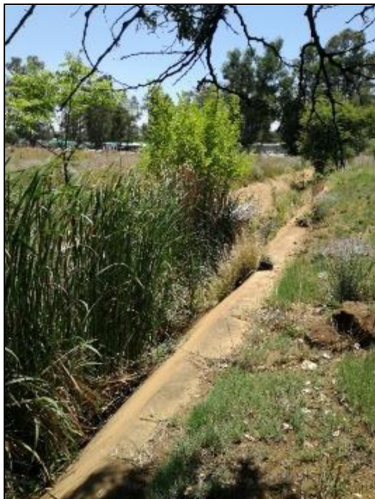
Figure 7: South side of channel also overgrown
