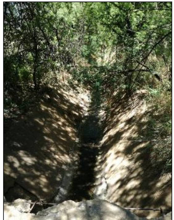
Figure 8: Cracks in Concrete
