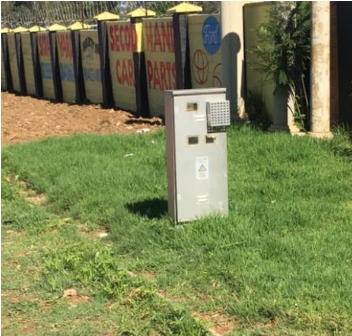
Fig 1. City of Tshwane meter box on site boundary
