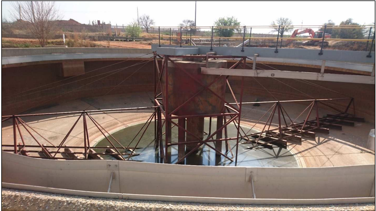
Figure 11: Fermenter bridge and scraper mechanism
