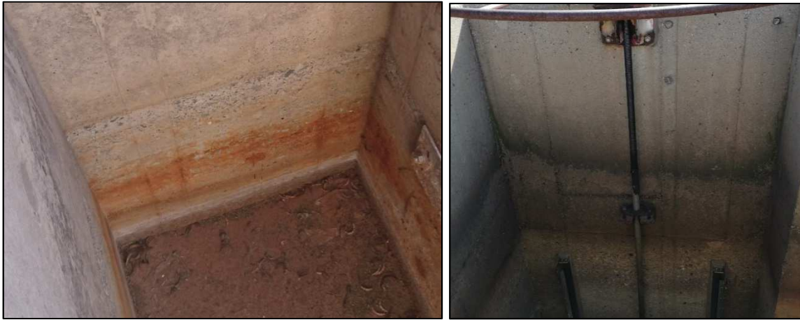
Figure 4: Deterioration of concrete inside PST division box
