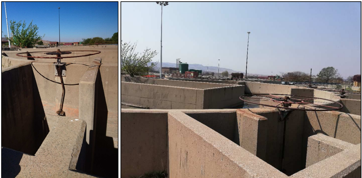
Figure 10: Sluice gates at the existing PST division box
