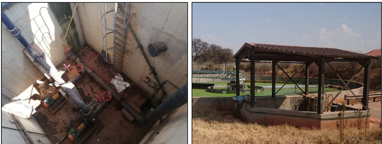
Figure 6: Pump station servicing PST 5
