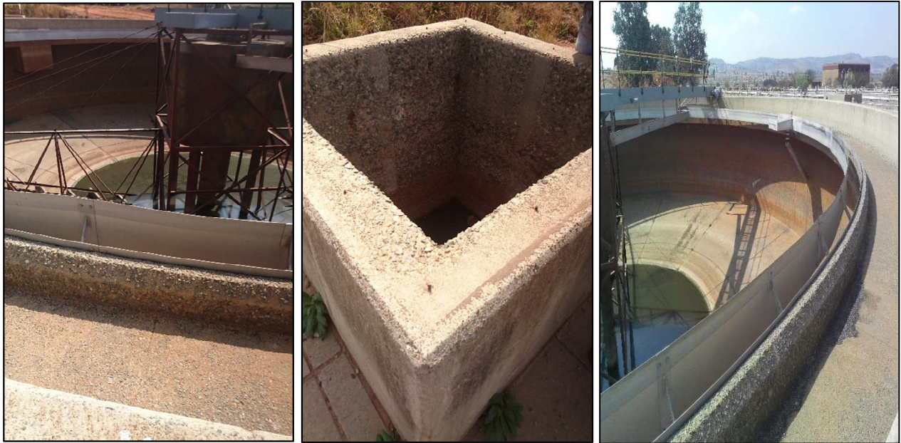
Figure 7: Deteriorated concrete in the Fermenter launder and Fermenter Outlet Box
