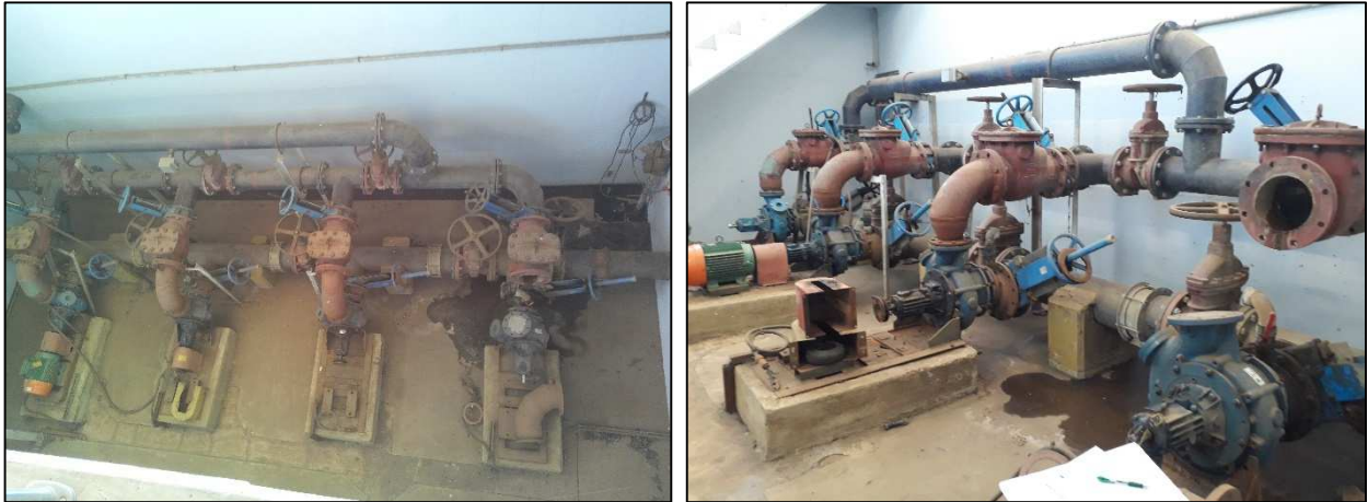
Figure 5: Interior of Pump Stations servicing PST 1 -4
