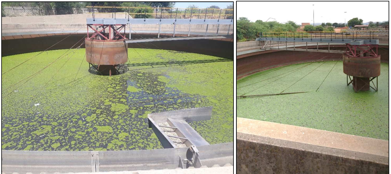
Figure 8: Bridge and scraper mechanism for PST 4
