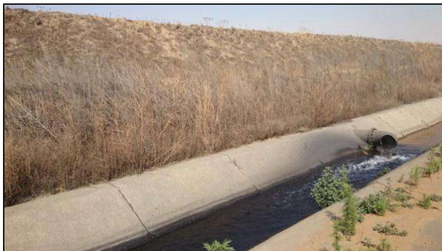
Figure 8.1: Trapezoidal channel collecting water from discard dump penstock outlets
