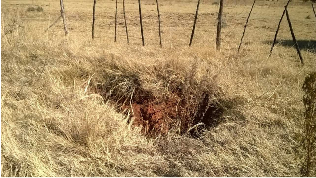
Figure 6 | Existing sinkhole at point 4 on Site 2 as shown in Figure 7
