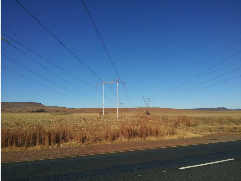
Figure 9 | Three 132 kV parallel distribution lines traversing Site 2 (view to the south with the R501 in the foreground)
