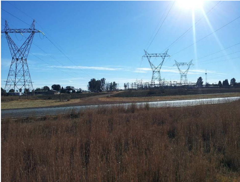
Figure 8 | Libanon Distribution substation located to the north of the R501, adjacent to Site 1 and opposite Site 2
