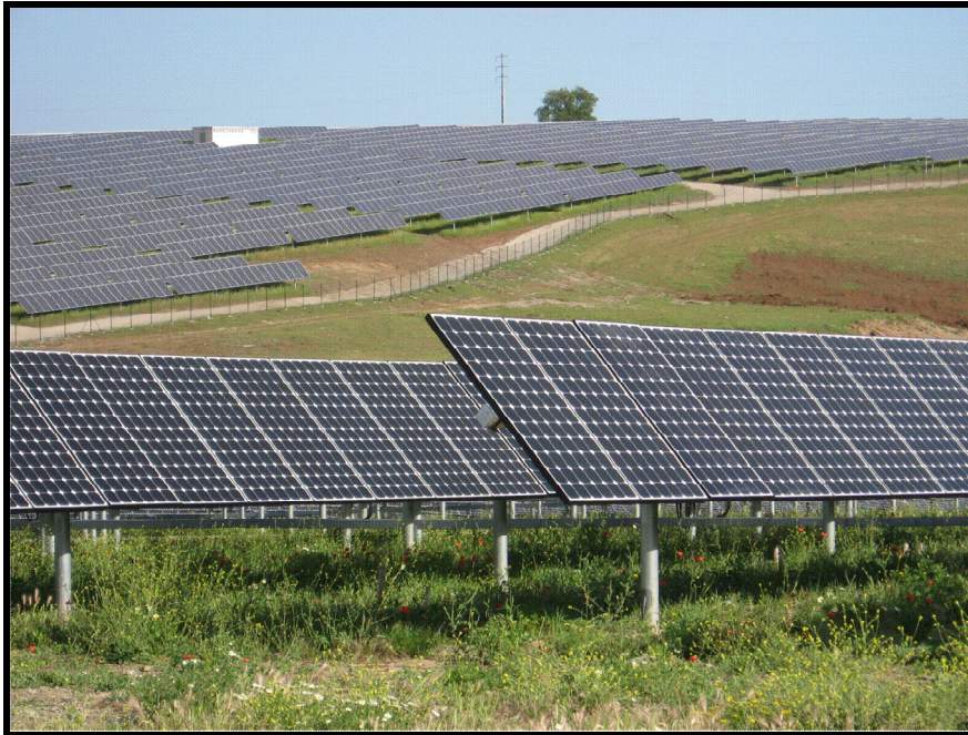
Figure 1.2: Stationary solar PV panels.
