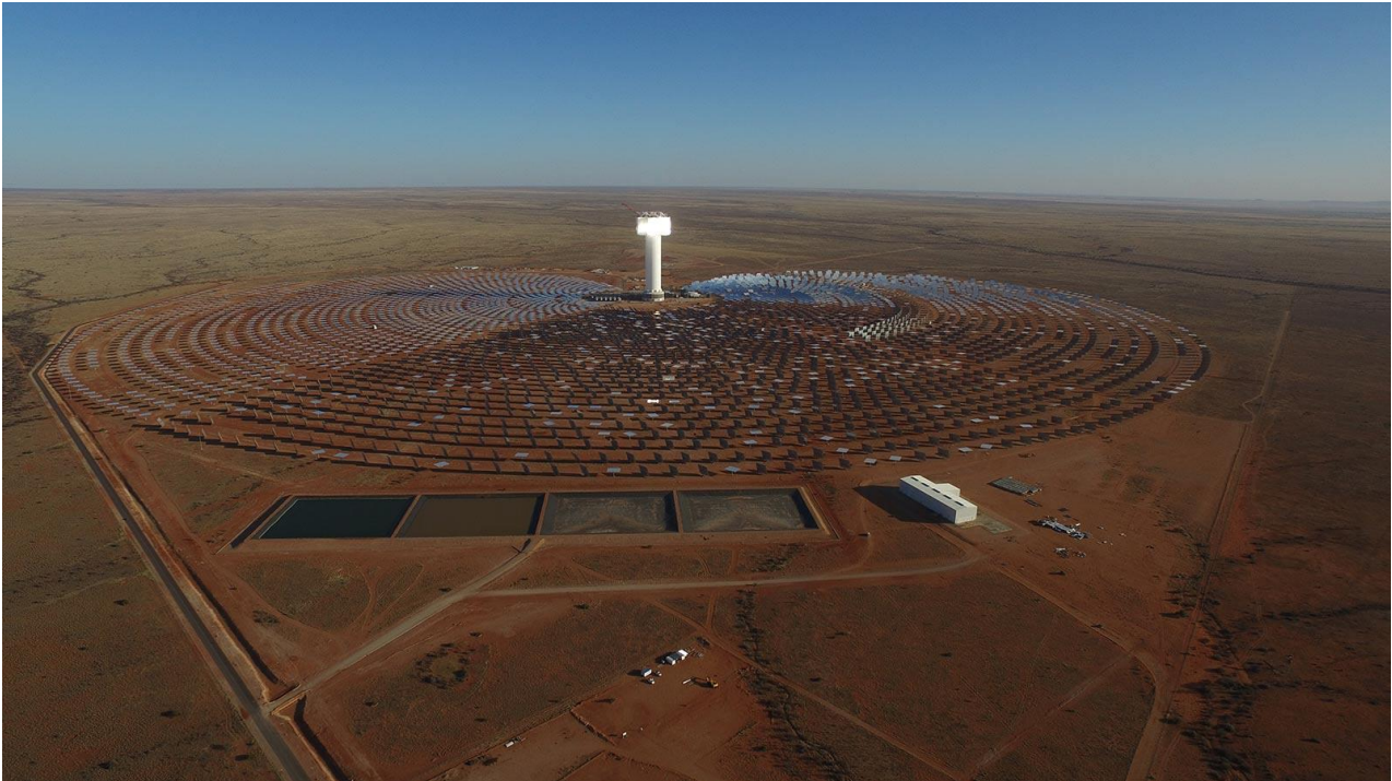
Figure 4.3: Operational Khi Solar One located in the southern corner of Portion 3 of the Farm McTaggart's Camp No. 453 (source: www.energy.org.za )
