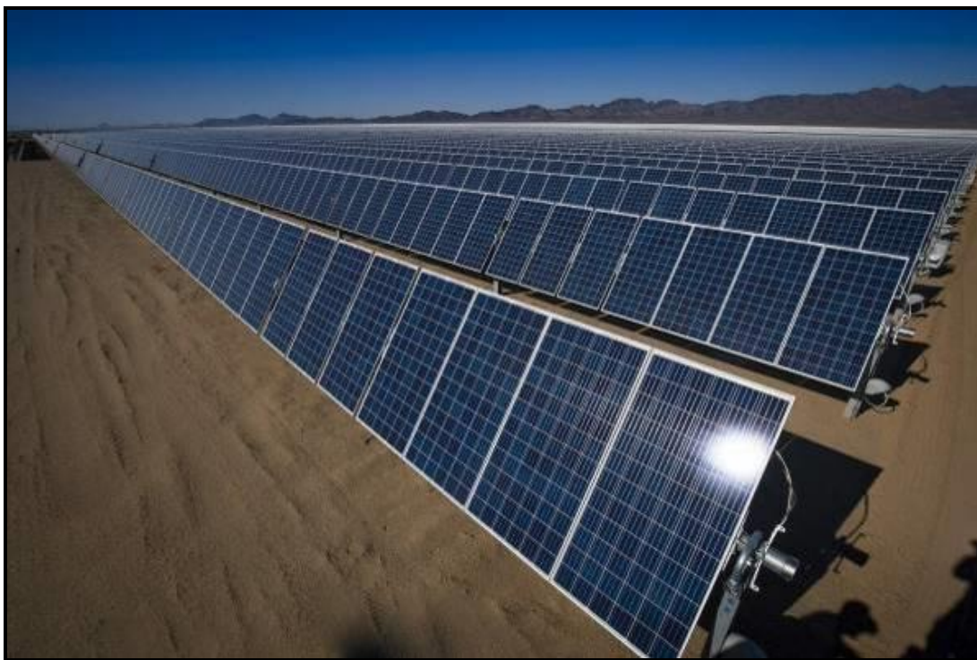
Photograph 1.1: Typical PV SEF facility
