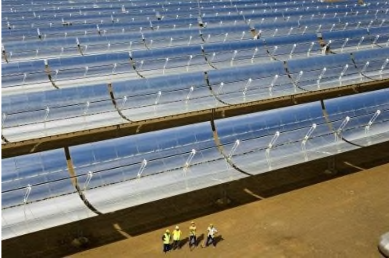
Plate 1, Existing Parabolic Trough Solar Field. (photograph extracted from solarhomes web site, http://www.jc-solarhomes.com )
