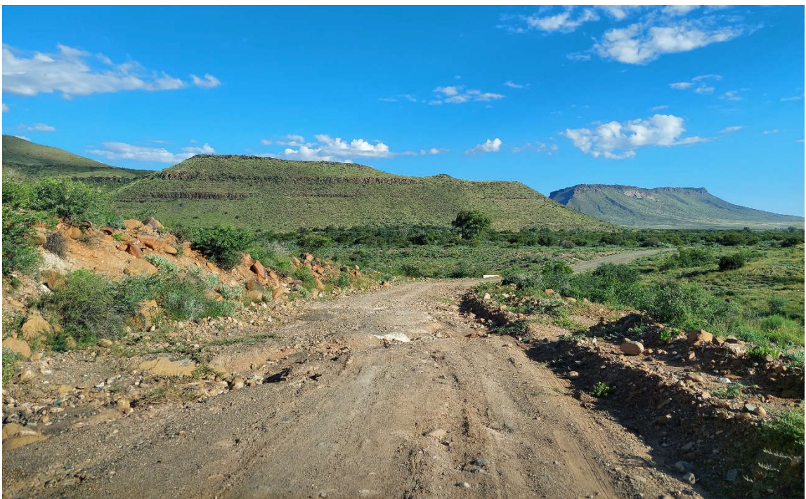
Photo 3-3: Poor condition of DR2383 due to lack of drainage infrastructure
