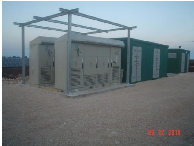
Figure 14 : Typical onsite substation
