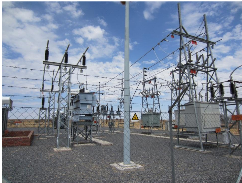
Figure 13 Schuitdrift Eskom substation
