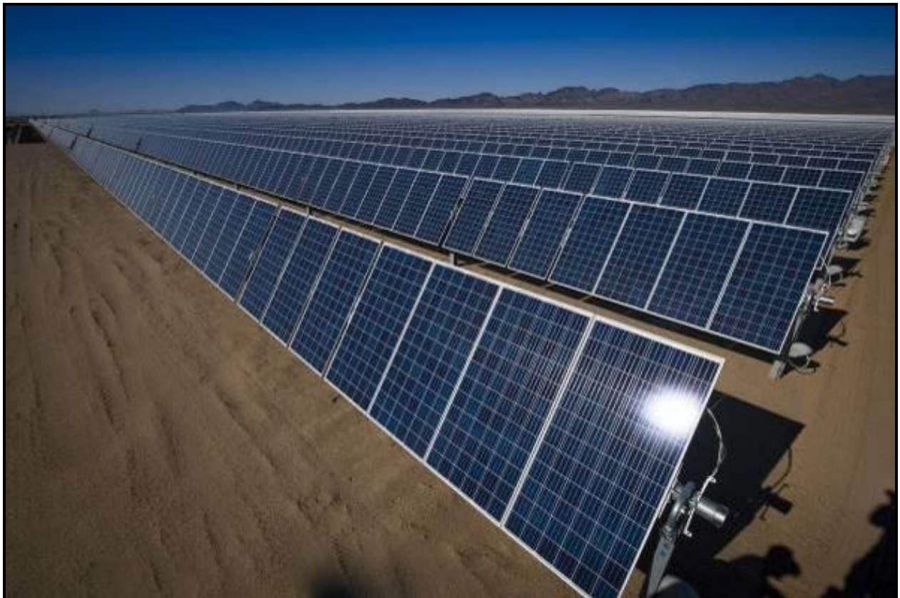
Photograph 1.1: Typical PV SEF facility
