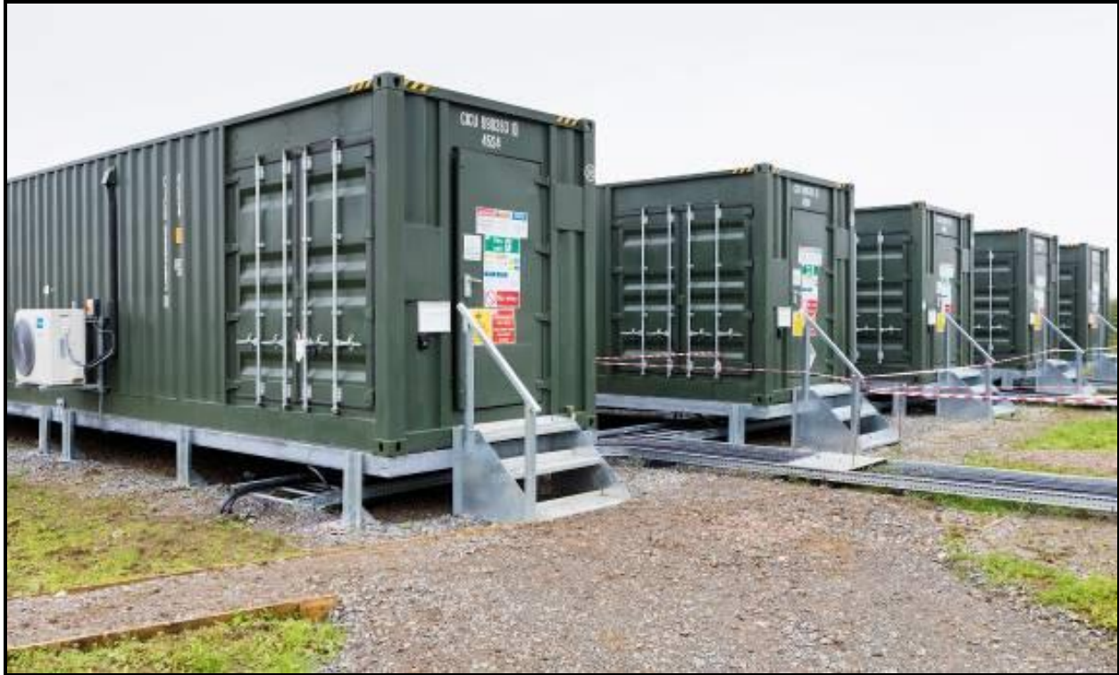
Photograph 1.2: Example of BESS located in storage containers
