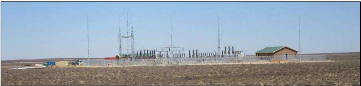
Photograph 2: Khobab WEF substation under construction, seen from, the Granaatboskolk gravel road, December 2016.
