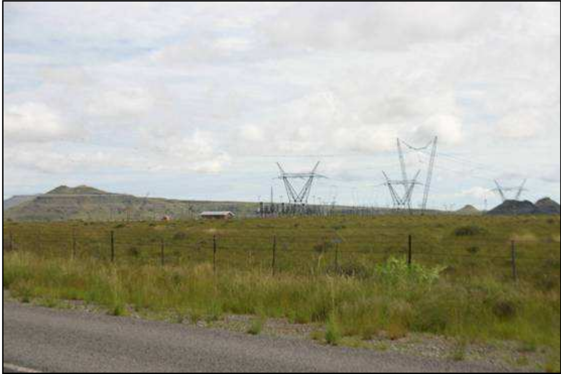
Figure 7: The Victoria Substation to the north-east of the site, adjacent to the R63.
