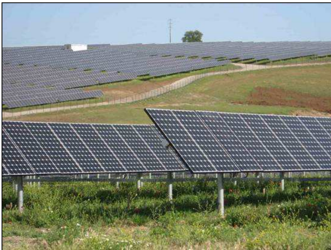
Figure 2: Photograph of typical Photovoltaic panels
