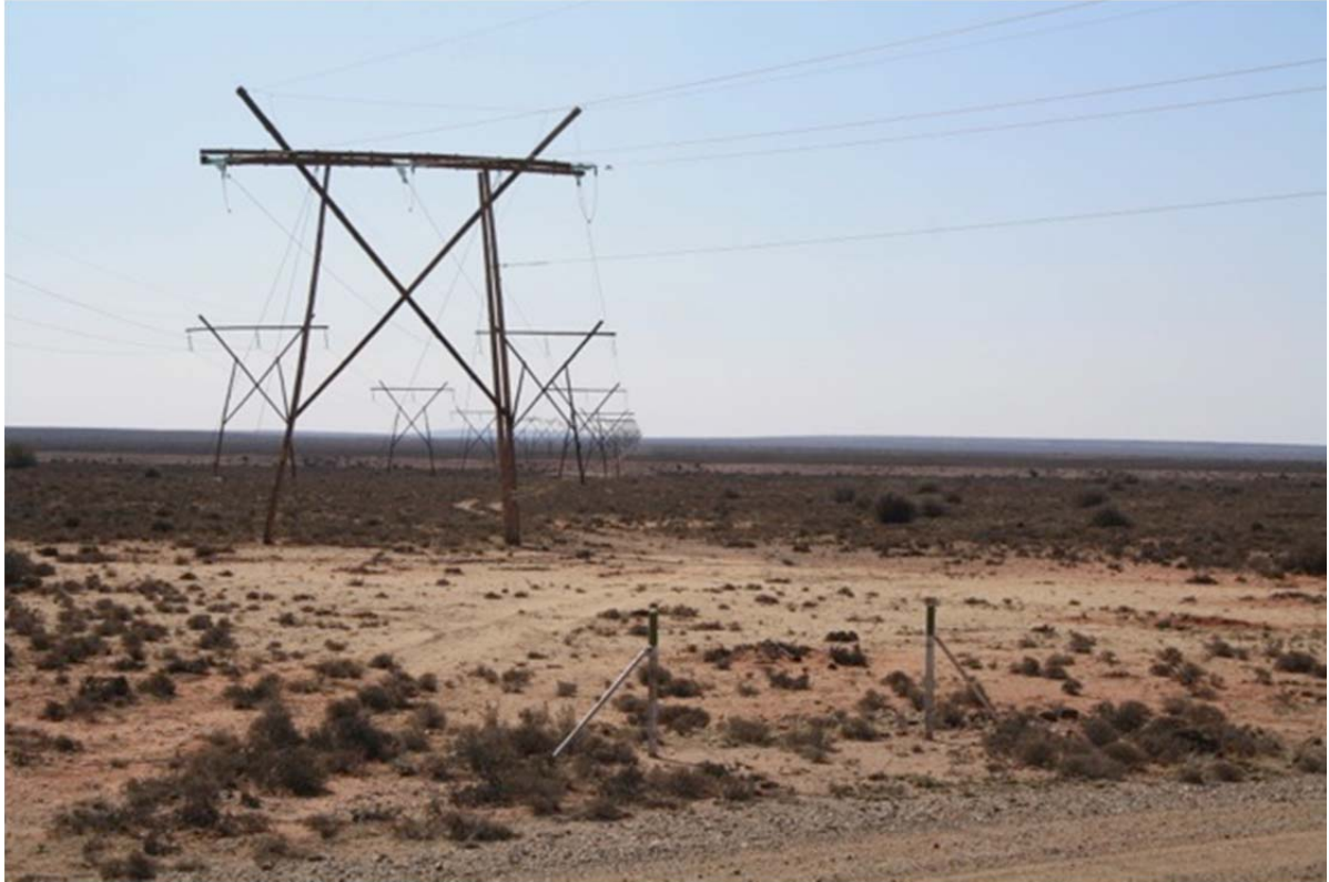
Figure 4: 132 kV powerlines traversing the study area
