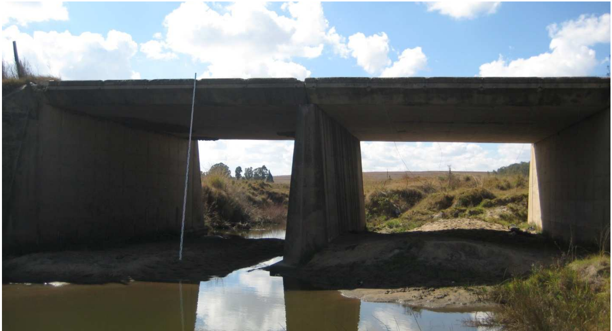
FIGURE 5-6: RIVER CROSSING OVER STEENKOOLSPRUIT MAIN CHANNEL NORTH-WEST OF SHAFT COMPLEX - FACING UPSTREAM (EAST)
