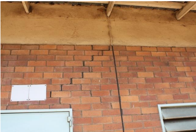
Figure 11: Example of blast induced damage.
