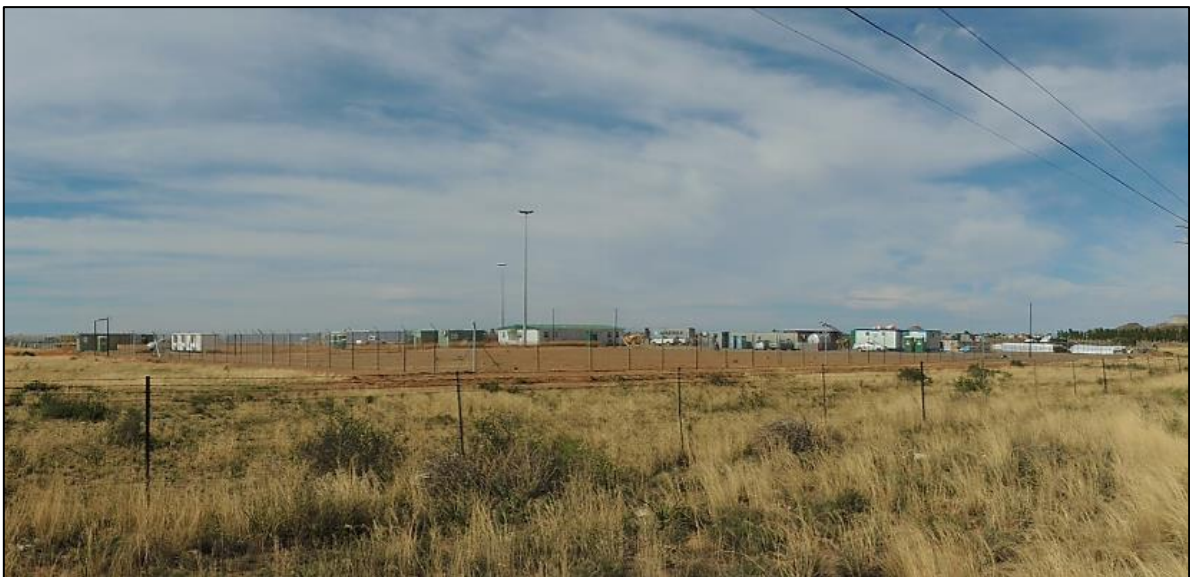
Figure 4. Typical construction site and laydown with fences (excluding overhead lighting) (Source: VRMA)
