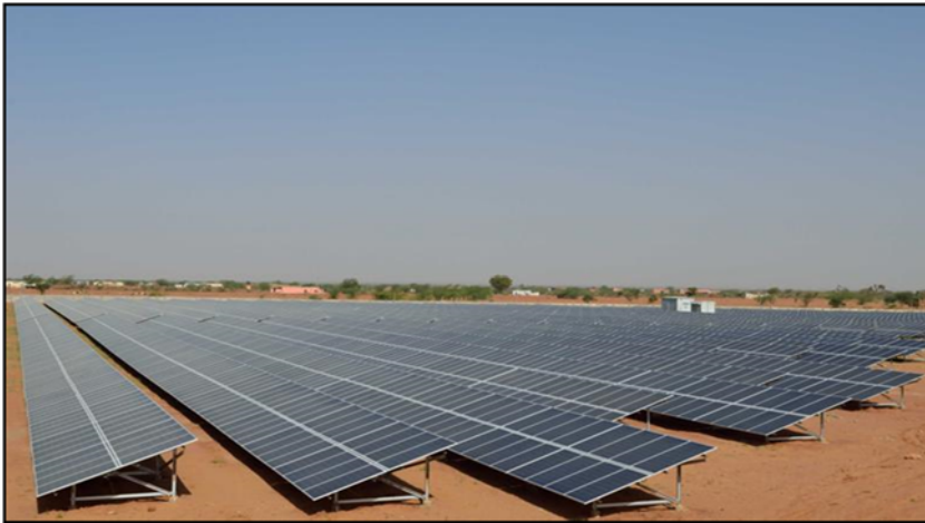
Figure 1-2: Example of PV Solar Power Facility's Tracker View 2
