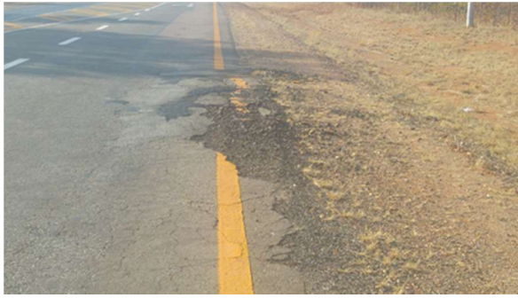
N1/D1021 intersection (pavement distress on N1)
