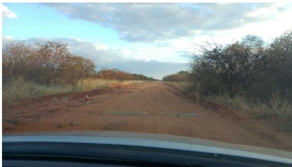
D744 - Exposed culvert
