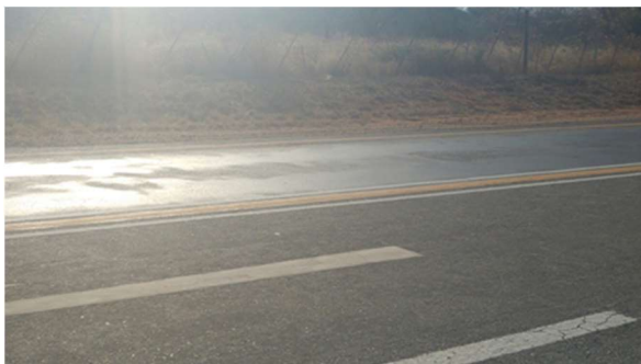
N1/D1021 intersection (bleeding road surface bleeding on N1)
