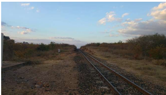
D1021 - Sight line to north at rail level crossing limited by narrow cutting and rail line geometry
