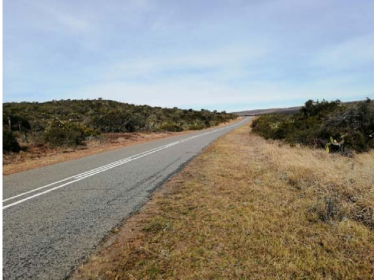
Figure 3 – Condition of Road MR00477 (R350)
