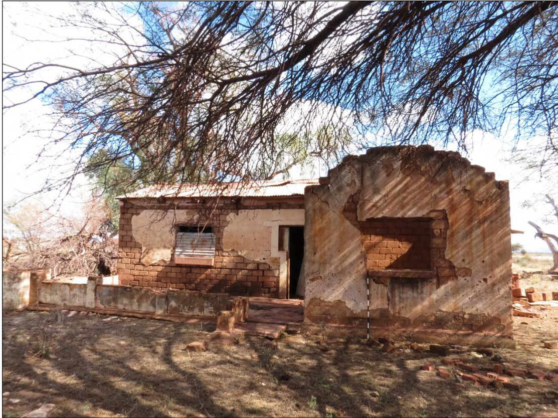
Figure 33 – Eastern façade of the dwelling showing the veranda (left) and stoepkamer (right)
