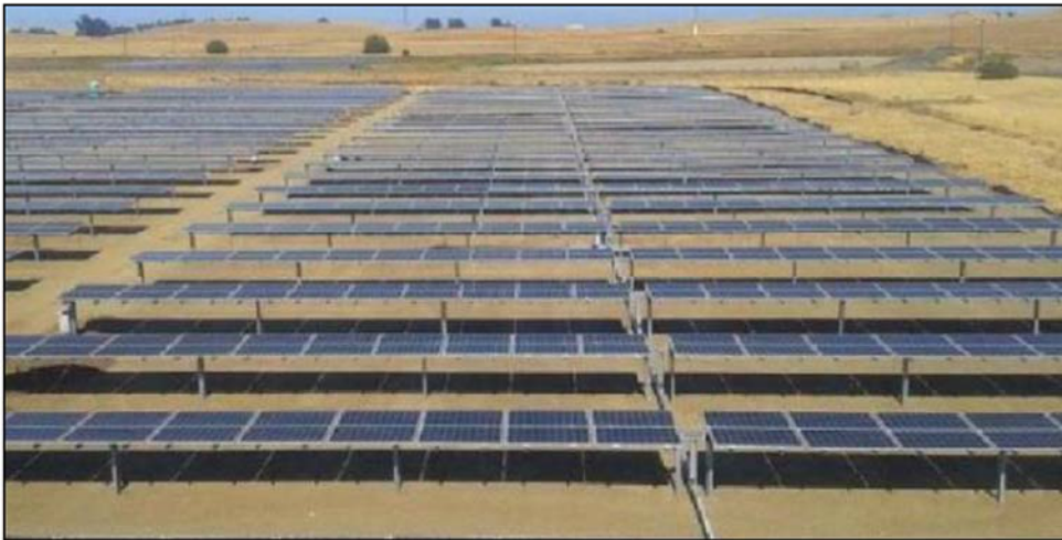
Figure 3: Example of PV solar power facility's tracker view
