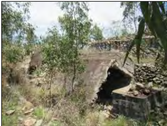
Figure 88: View of large ruined stone and cement structures
