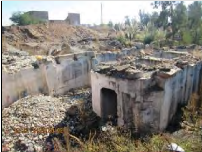
Figure 56: Site WW-003, view of remains of structure that could have held explosives
