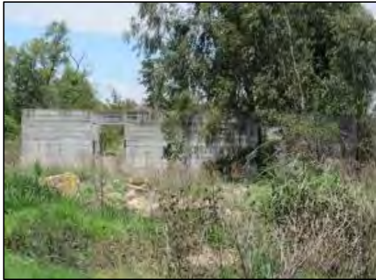
Figure 90: View of ruined concrete structure
