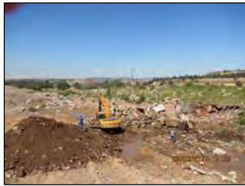
Figure 24: 11 Shaft Main Reef Pit area, showing illegal mining activities
