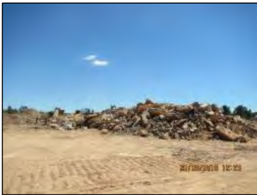
Figure 23: 11 Shaft Main Reef Pit area, showing the building rubble from demolished mining structures
