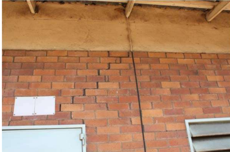
Figure 7: Example of blast induced damage.
