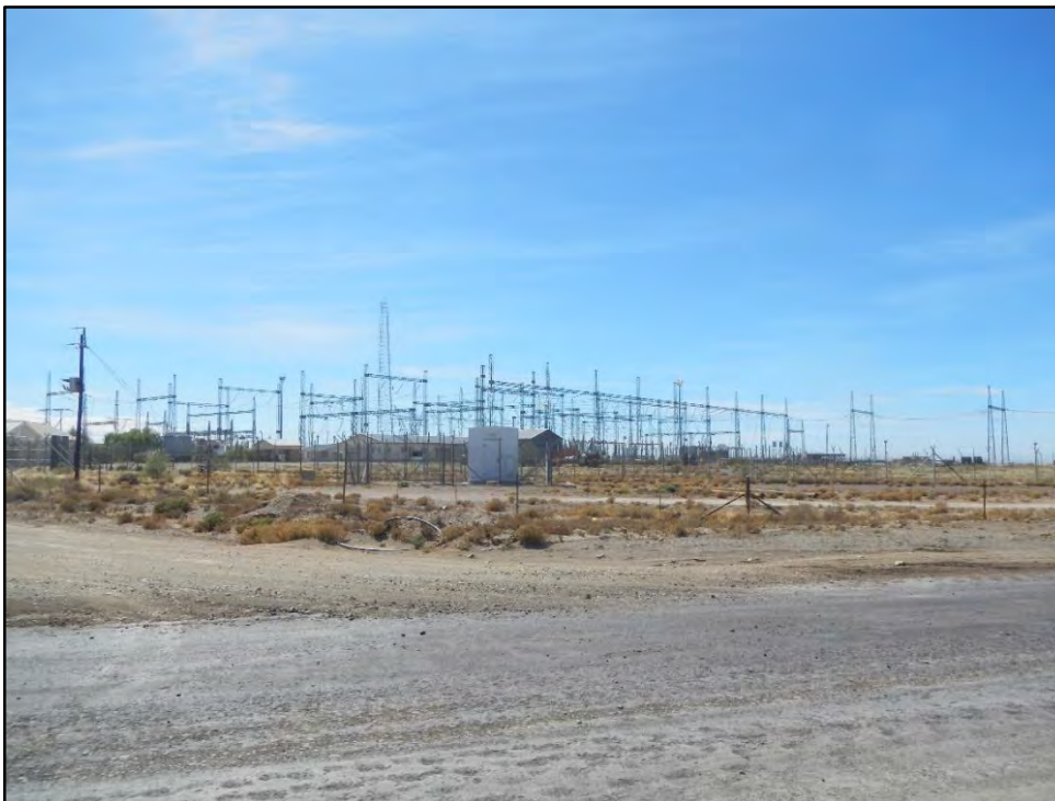
Figure 17: View of Helios Substation
