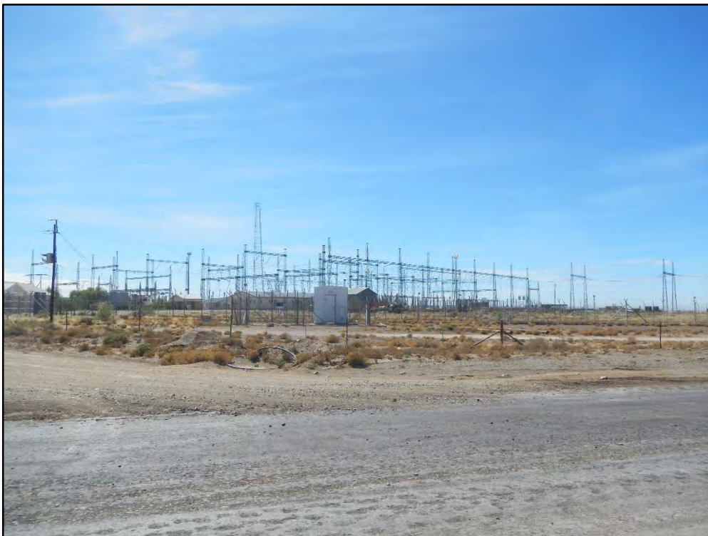
Figure 17: View of the Helios Substation.
