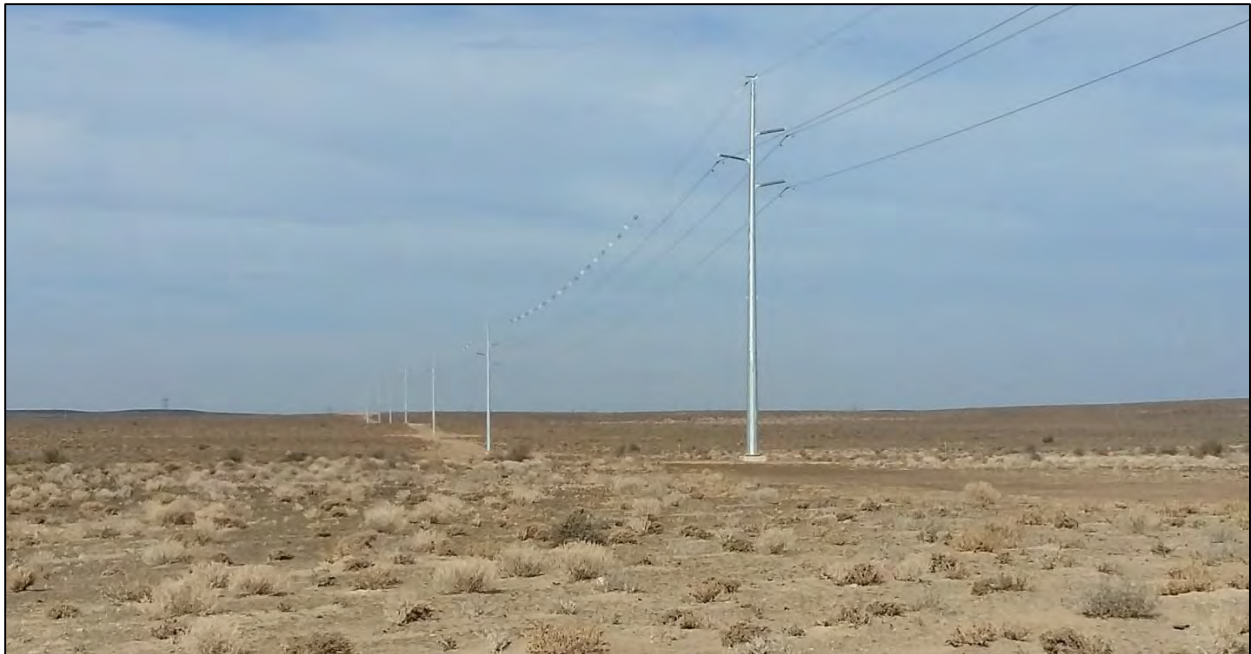
Figure 1. A section of the 132kV grid connection for the Mainstream Khobab Wind Energy Facility, showing the type of infrastructure to be used and the associated footprint.
