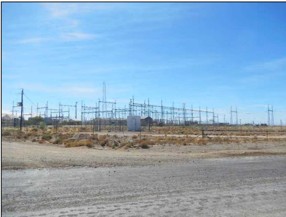
Figure 17: View of Helios Substation.
