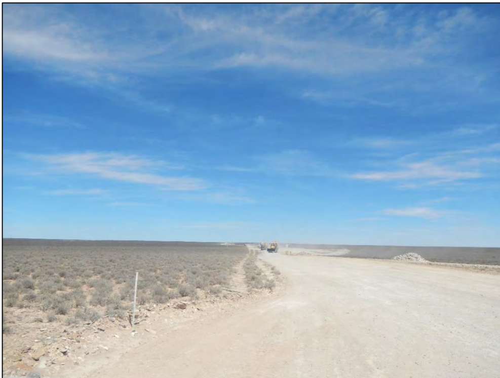
Figure 22: View of the construction activities associated with the proposed Khobab Wind Farm. During the time of the in-field investigation it was noted that this wind farm was still in the early stages of construction and no turbines had thus been erected.
