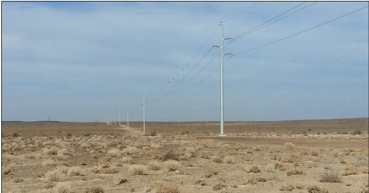
Figure 1. A section of the 132kV grid connection for the Mainstream Khobab Wind Energy Facility, showing the type of infrastructure to be used and the associated footprint.
