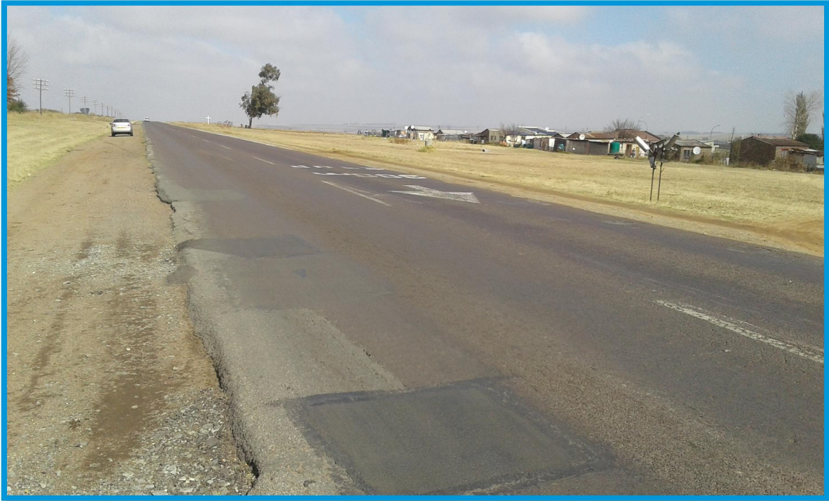
Photo 19: R547 towards Kriel – Edge Breaks and Localised Patching
