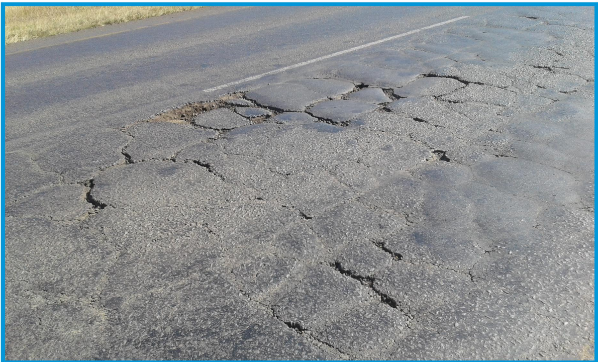
Photo 10: Surface Cracks and Developing Potholes
