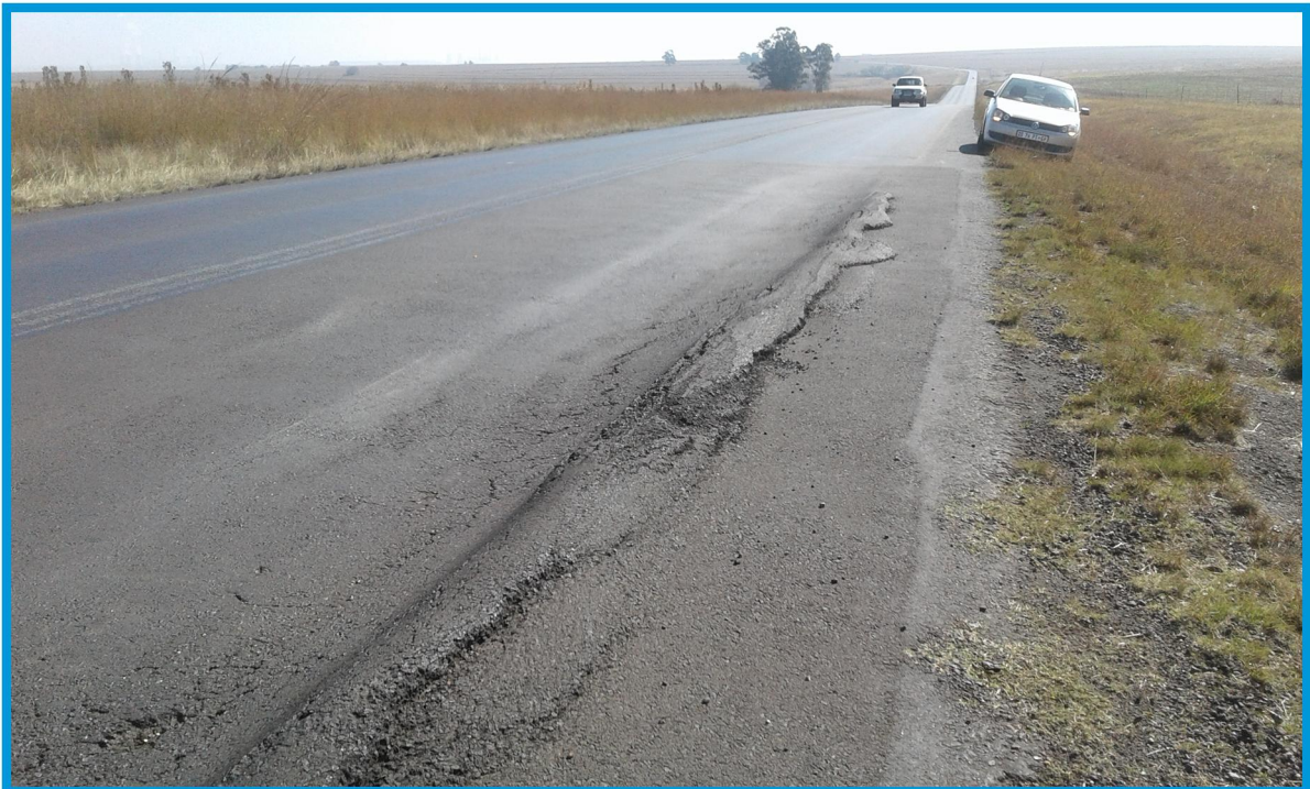
Photo 8: Rutting and Shoving of Asphalt – R545 East of Kriel
