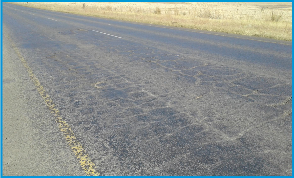
Photo 11: Pumping; Surface Cracks and Developing Potholes
