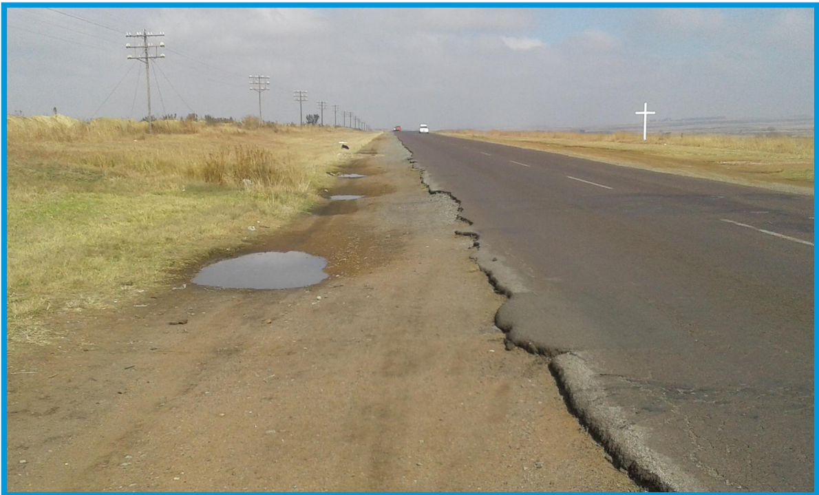
Photo 20: R547 towards Kriel – Edge Breaks Including Patched Edge Breaks
