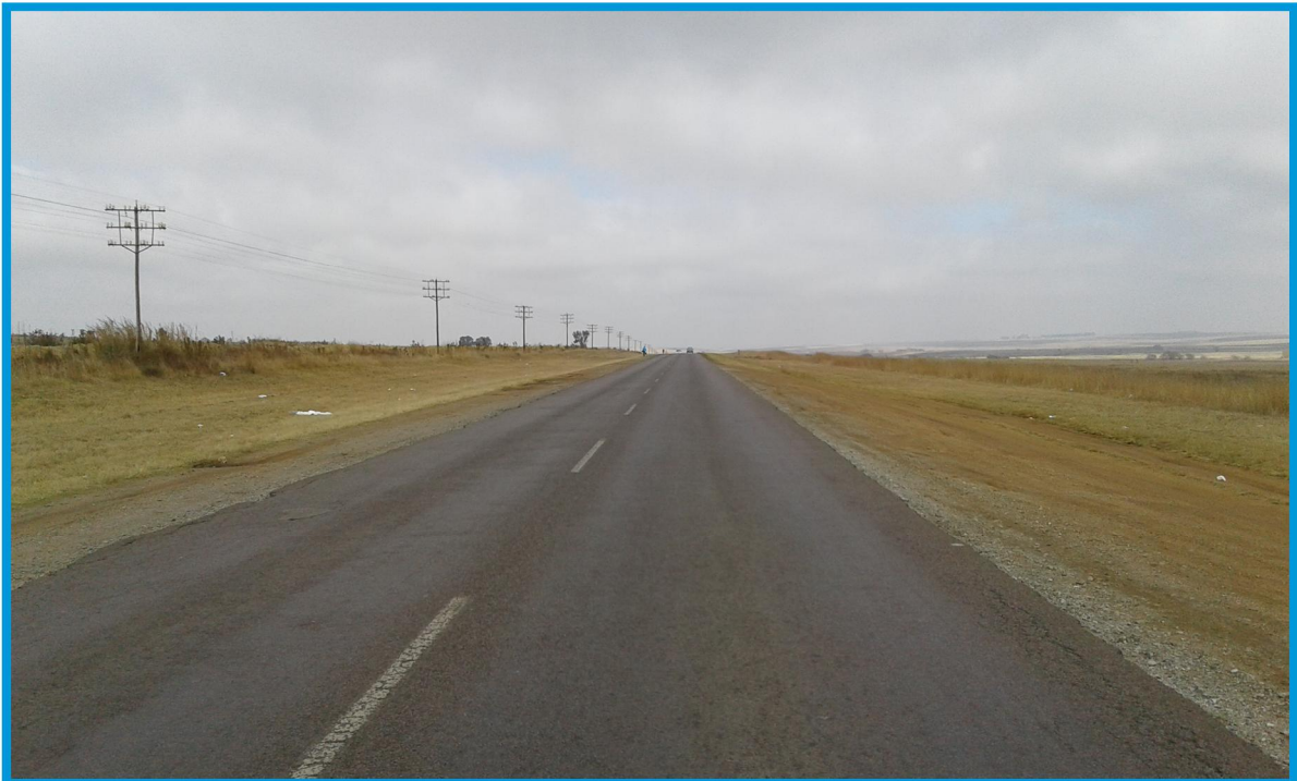
Photo 18: R547 towards Kriel - General Road Condition
