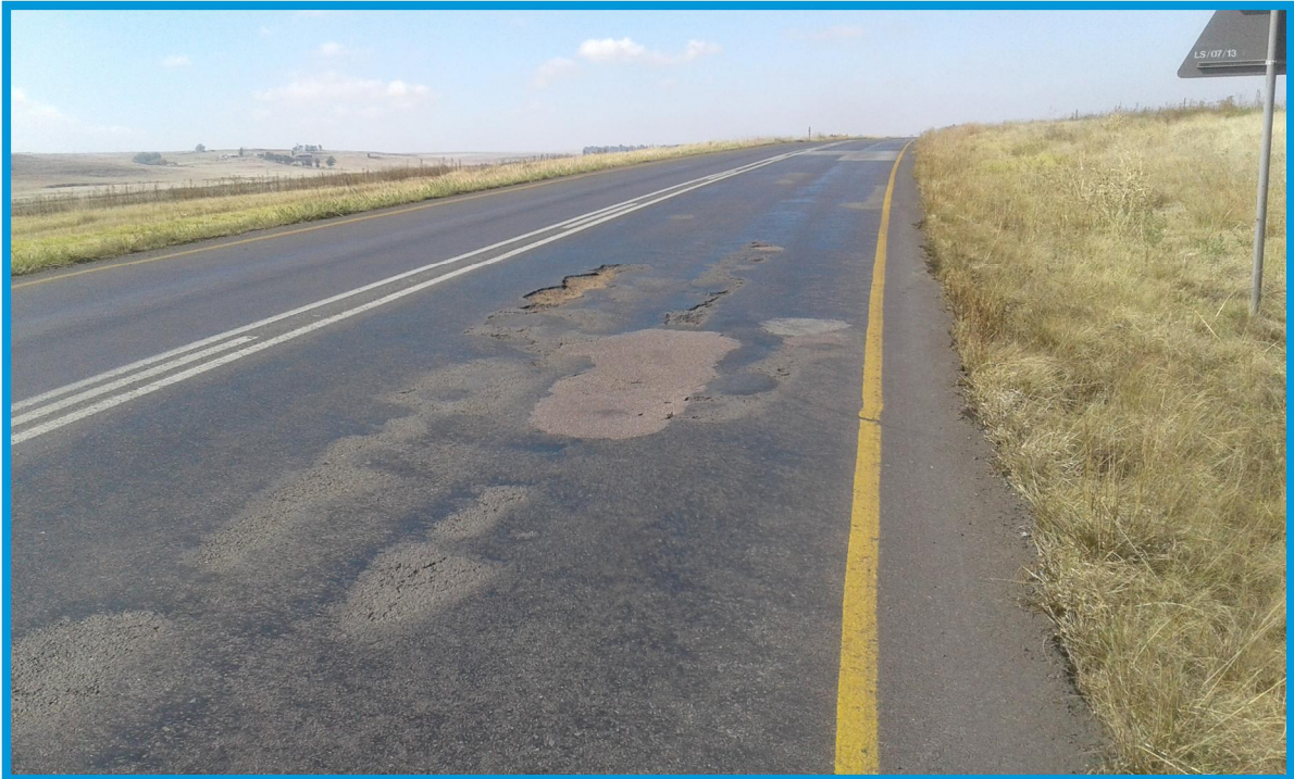
Photo 7: Surface Failure Leading to the Formation of Potholes (incl. Patching) – R545 East of Kriel
