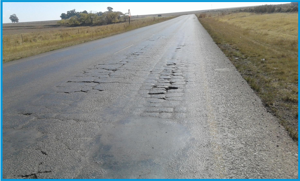
Photo 9: Surface Cracks and Developing Potholes
