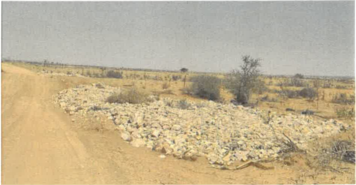
Figure 12 Riprap in eroded areas
