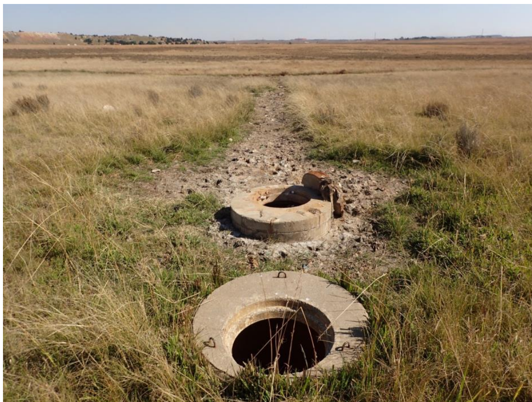
Figure 7-1: Open sewage cover with signs of flow into the Saalkspruit
