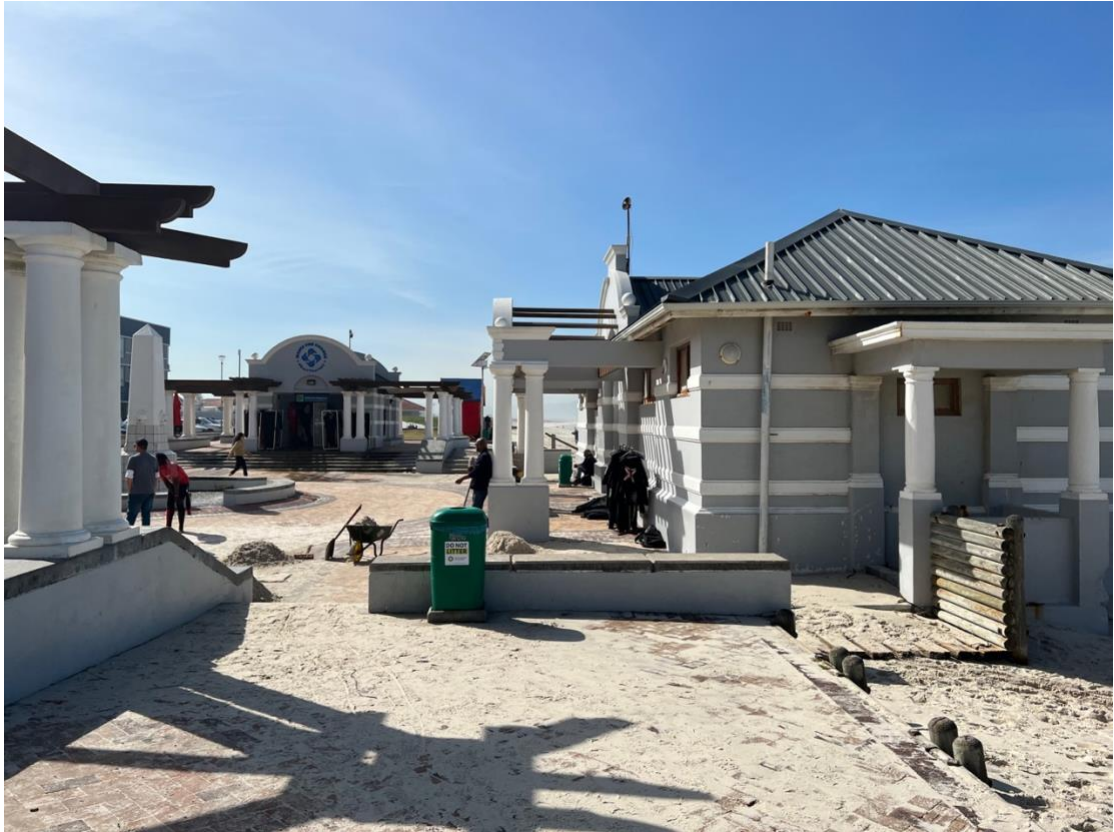
Another North-East facing view of the site. This is the central area of the site. The ablution block (visible on the right) will be moved back (landward) from the beach. The current sea wall is visible in the foreground of the photo.
