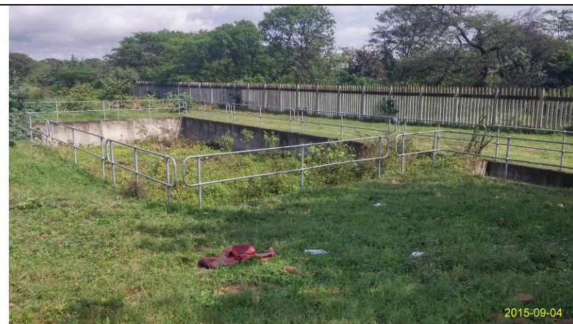
Looking south-west. Photograph taken near Position 3. Defunct leachate collection infrastructure.
