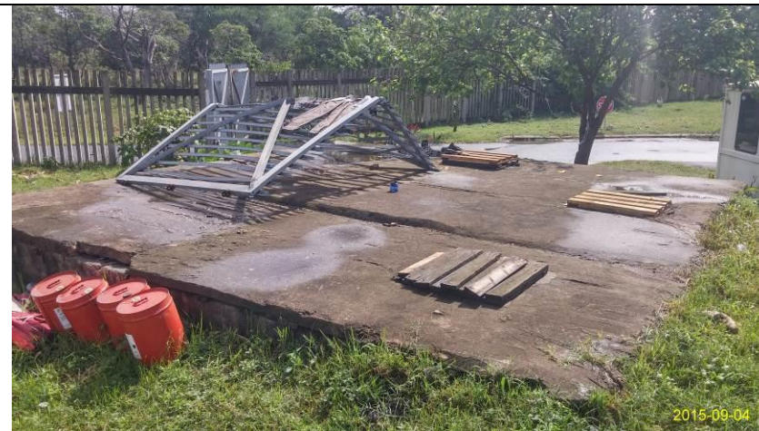
Looking west. Photograph taken near Position 3. Defunct leachate collection infrastructure.
