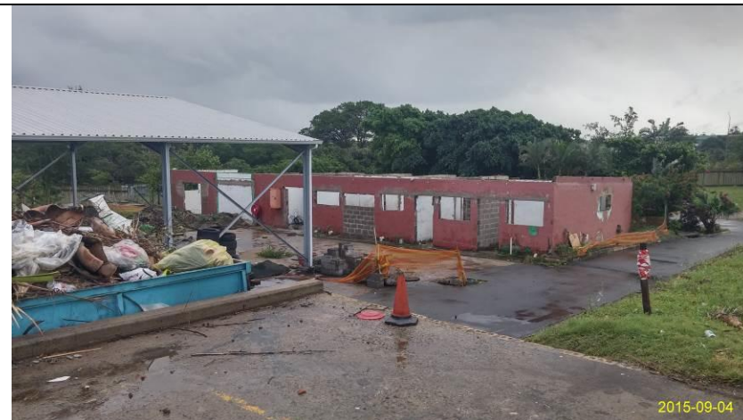
Looking north-west. Photograph taken near Position 1. Admin block, plans are underway for its rebuilding.
