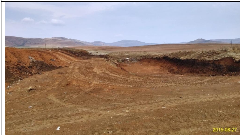
Looking south-west. New unlined trench. In the distance beyond the fence is the old landfill area. Photograph taken between Positions 2 and 3.
