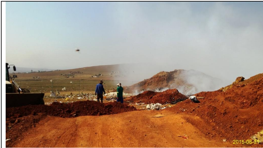
Looking east. Waste sorters working at active landfill area, near the fire and TLB. Photograph taken near Position 4.
