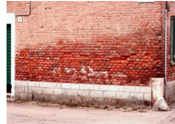
Tide marks – Damp patches
