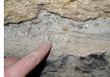
Brittle, sandy plaster
