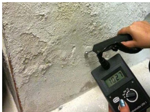
High damp meter readings
