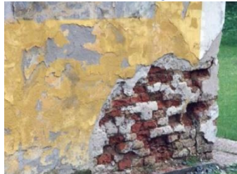
Destroyed building fabric
