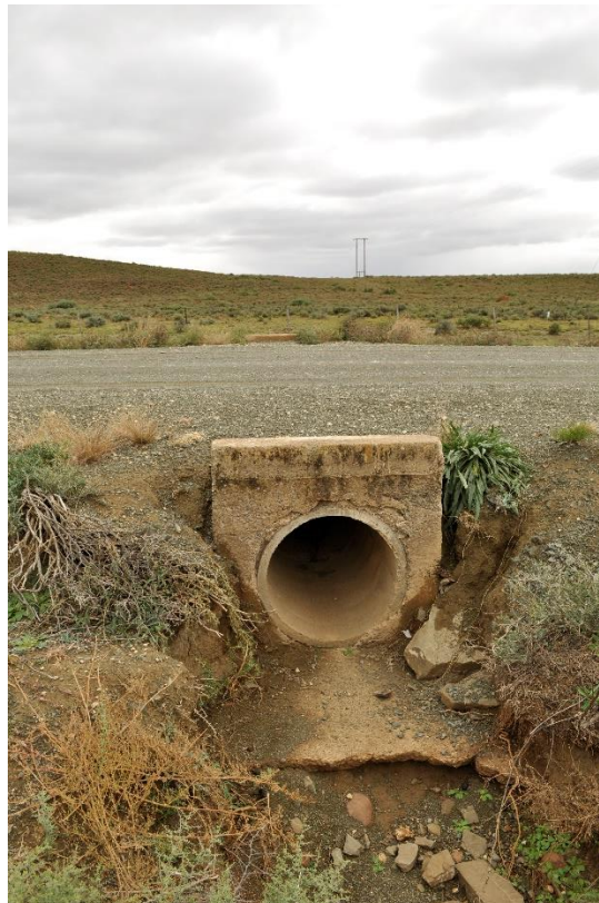
Plate 2: A typical water course observed within the study area, where the potential exists to improve the current state of flows and erosion protection
